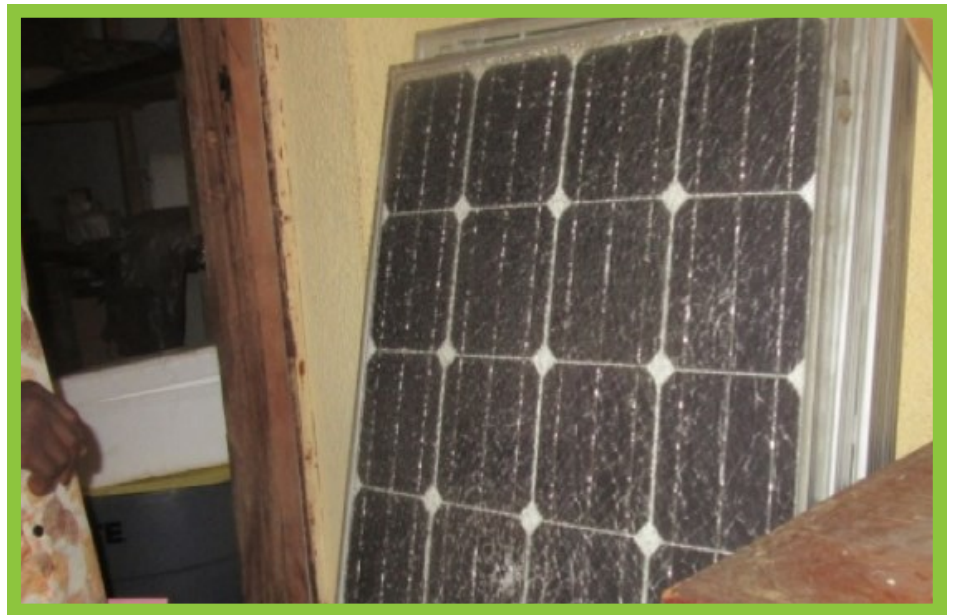
Three damaged solar panels awaiting replacement at the Walikale Hospital [Photo: Pact]
