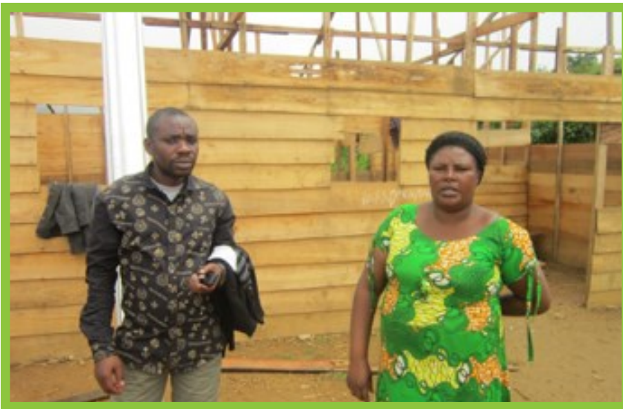
Nurse Valéry Rubona and president of the local health and development committee Furaha Baseme Nnagarhi supervising construction of the health centre [Photo: Pact]
